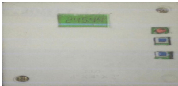
Fig. 5 Programmable protective device indicating over voltage condition
